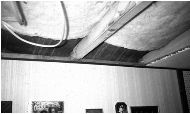
Figure 10-6 Incomplete Roof Insulation
