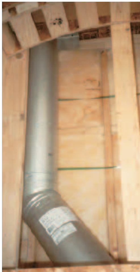
Figure 4. Batts behind manufactured fireplaces are strapped in place so they won't sag or droop. Kraft-faced batts aren't used because the facings are combustible.
