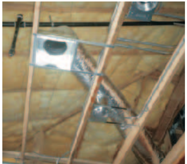
Figure 10. This example of a low-pitch cathedralized attic roof shows how the ductwork is brought within the conditioned space. Batts fit neatly into the roof-plane cavities, avoiding the need to make complicated cuts and fits around the can lights and other ceiling penetrations.
