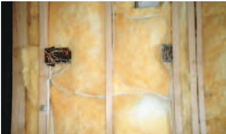
Figure 1. Irregular stud cavities, wiring, and other obstructions in a wall like this make it harder to cut and fit fiberglass accurately. Dark lines and visible stud shoulders in this wall indicate a hurried job.
