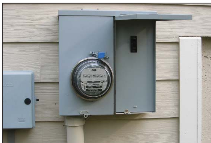
Figure 11.15. External Power Shutoff and Meter
