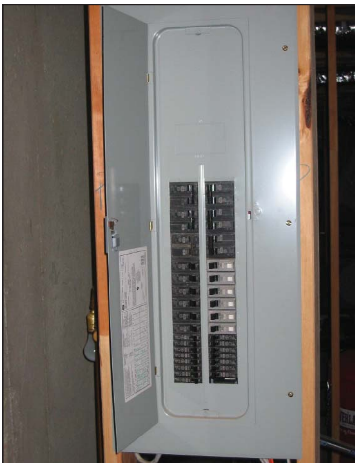
Figure 11.14. 200-Amp Service Box
