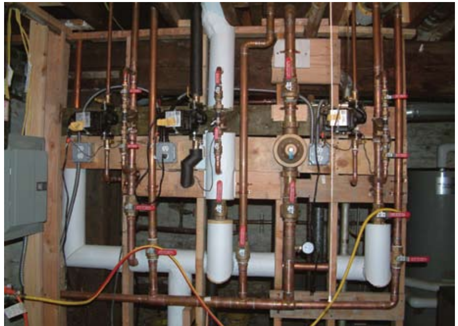
■ Figure 2. Photo shows three demand-controlled pumping systems, one for each wing of 12 units in a 3-story apartment building in San Francisco, CA, during major renovation. The pump for each wing is activated by a flow switch. Each unit is sub-metered for both hot and cold water and has its own demand-controlled pump activated by time-delayed motion sensors. The three main pumps each run less than 1 hour per day, and the pumps in each unit run about 15 minutes per day.
