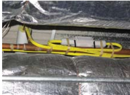
■ Photo shows a junction between two sections of self-regulating electric heat trace. The heat trace is mechanically strapped to the pipe. You can see 3/4 inch wall thickness insulation on the 3/4 inch pipe in the background. Source: Craig Drake, Tyco Thermal.
