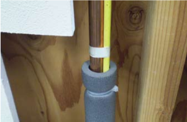
■ Figure 4. Photo shows self-regulating electrical heat trace strapped to the copper pipe and wrapped in insulation.
