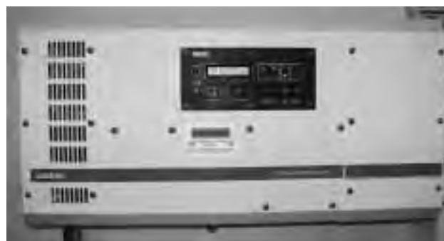
This inverter/controller converts direct current to alternating current, controls the charging of a bank of batteries, and manages a net metering connection with the electrical grid.
